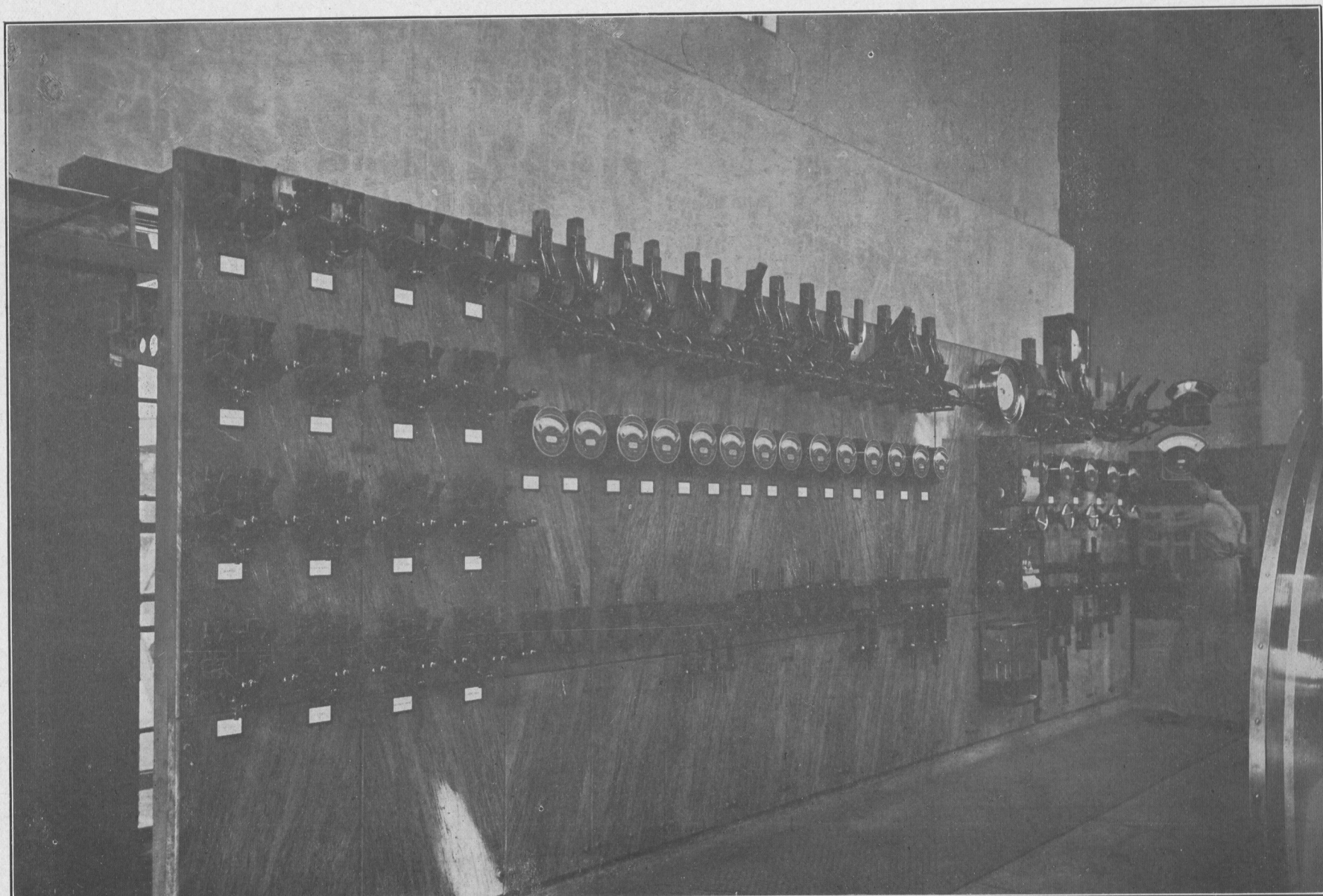
VIEW OF SWITCHBOARD
