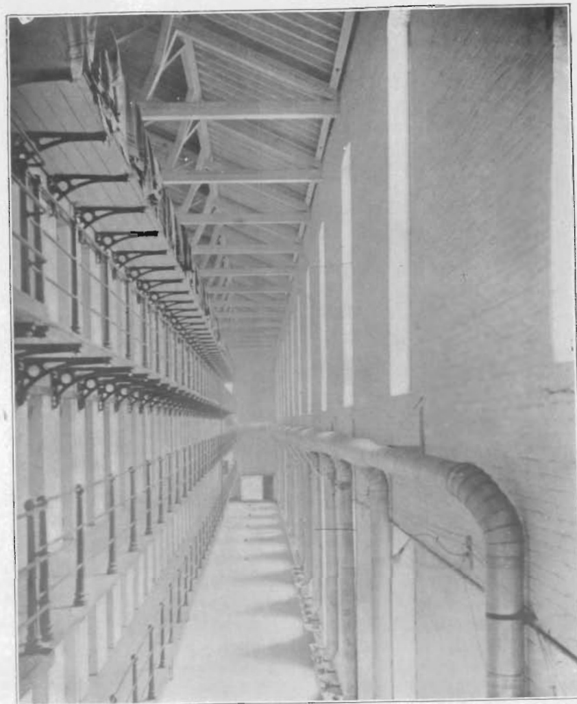
HEATING PIPES IN CELL-HOUSE CORRIDOR, INDIANA STATE PRISON.
